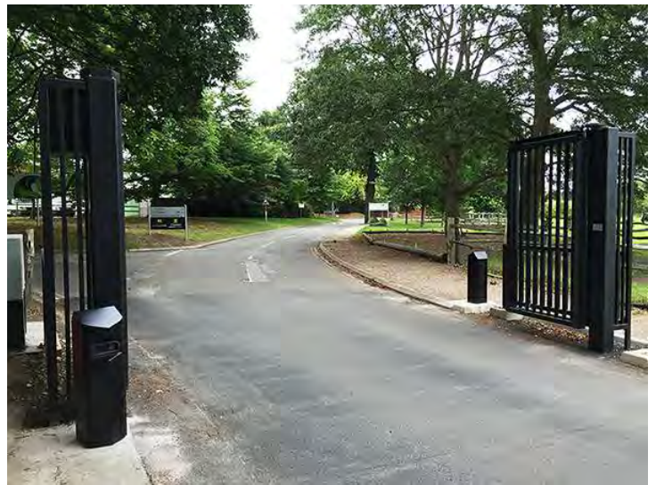
Two RoadWolf ANPR Bollards were installed to log the details of any vehicles attempting to gain entry or exit the site out of hours.
